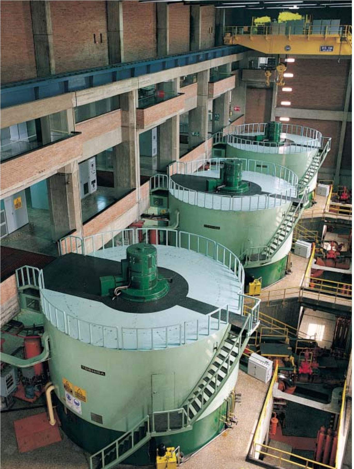
POWER HOUSE OF LA HUACA HYDROELECTRIC POWER PLANT, COLOMBIA
