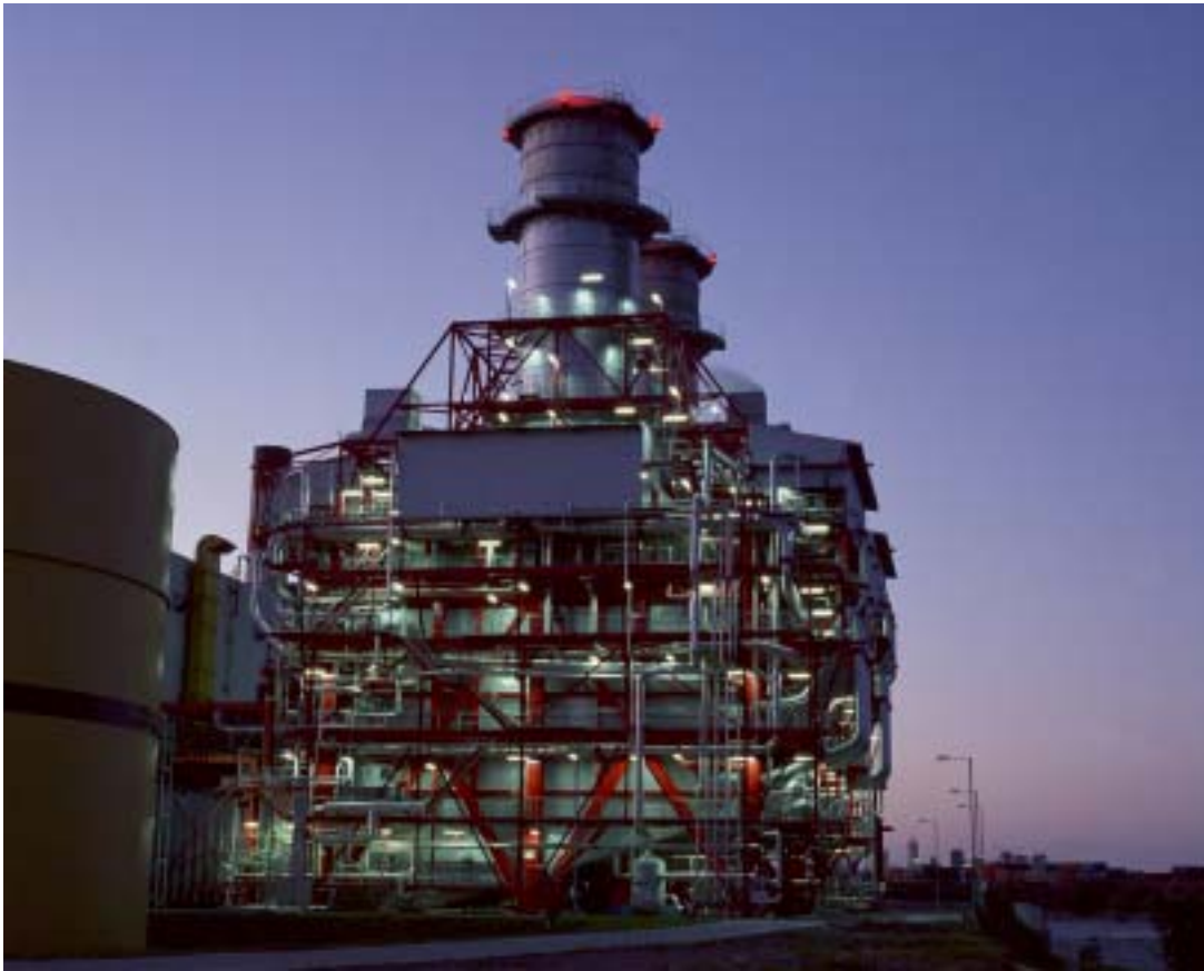
CENTRAL COSTANERA S.A.'S NATURAL GAS COMBINED - CYCLE POWER PLANT, ARGENTINA
