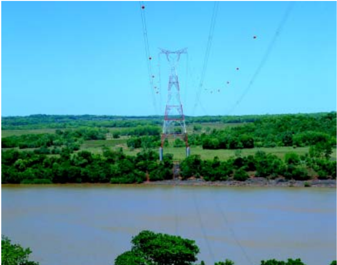
CROSSING OF PARAGUAY RIVER, CIEN POWER INTERCONNECTION ARGENTINA-BRAZIL
